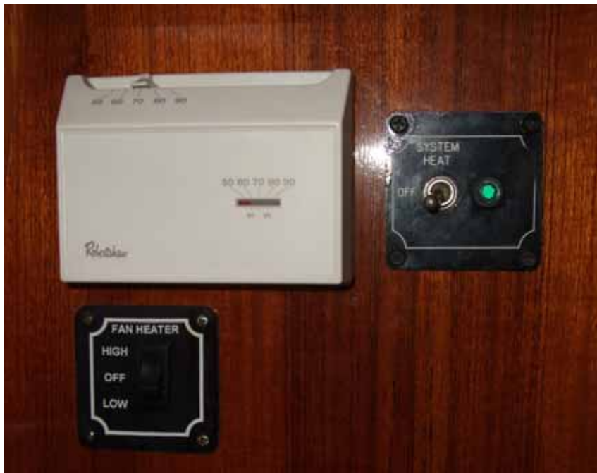
Nav station heater control: thermostat, on/off, main salon fan control
