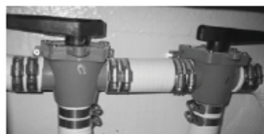
Gravity Drain Holding Tank
