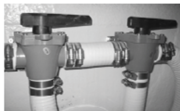
Into Holding Tank
