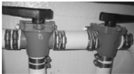
Gravity Drain Holding Tank
