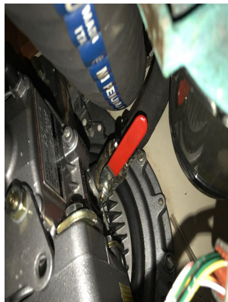
Raw Water Intake Valve feeding Sea Strainer (shown open). Access From side panel of engine compartment.
