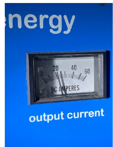
Charger (indicating 20A output)
