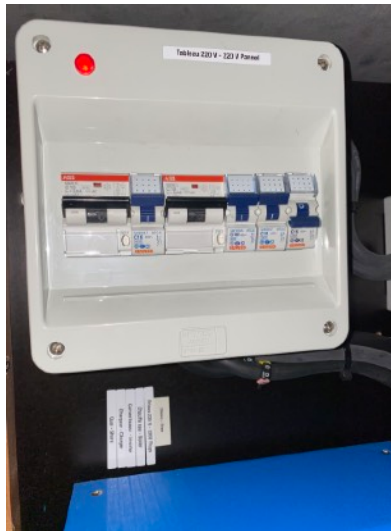
220v panel (indicating everything on except 'not-used')
