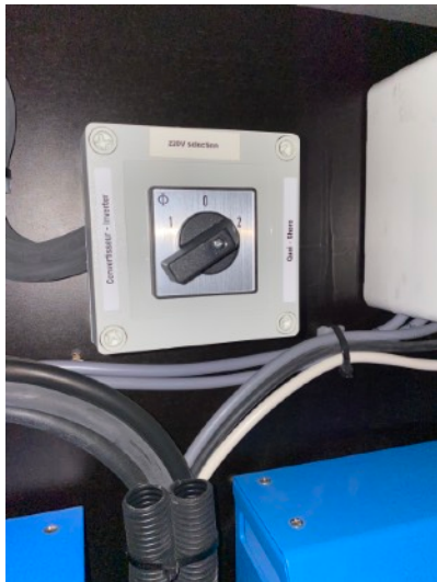
220v selector (showing shore power position)
