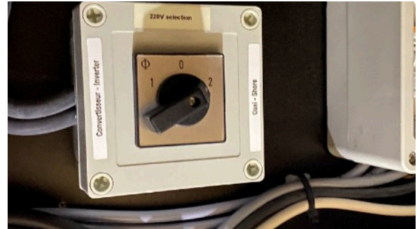
AC Bus Source Selector Switch
