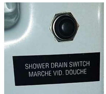
Sump pump switch in aft head.
