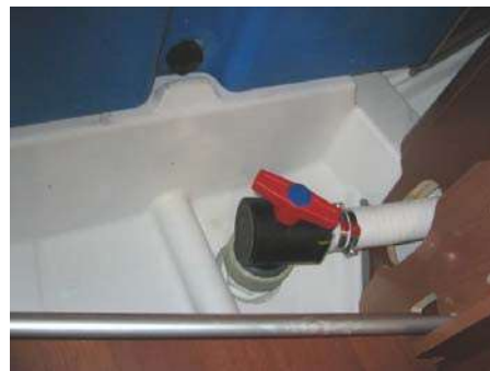
Forward head overboard discharge valve – located in forward cabin next to storage compartment under bunk; the compartment has been removed for easier access.
