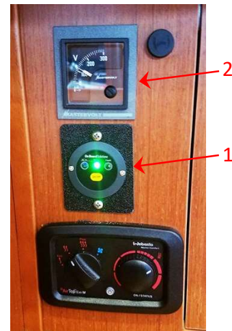
Inverter controls: ON/OFF Switch (1), voltmeter (2).
