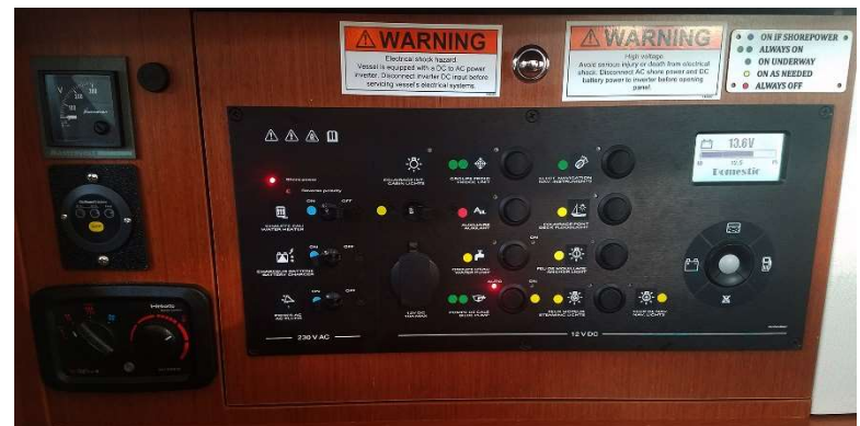
Electrical Panel – AC controls on the left, DC controls in the middle; toggle switch and LED on the right are used for checking battery charge and tank levels (fuel, water). Inverter & heater controls are on the far left.
