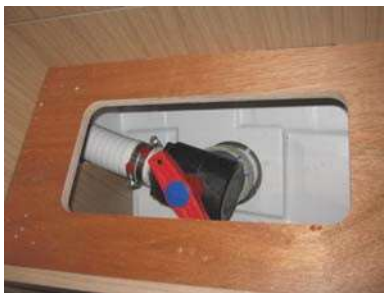
Aft head overboard discharge valve – located in starboard cabin under access panel in front of hanging locker.
