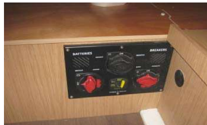
Battery switches – aft port cabin.
