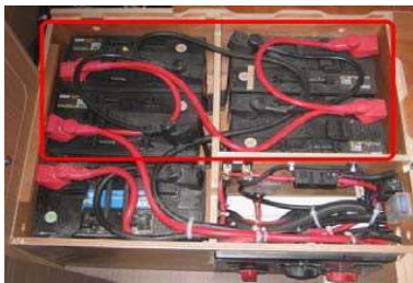
Battery bank – aft port cabin.
